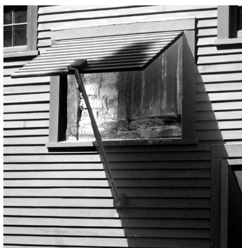
A hatch in the Coffin House exterior has been raised to show features of wall construction. This is an example of HNE's efforts, beyond restoration and caretaking, to enhance understanding of the historic homes under its care.
